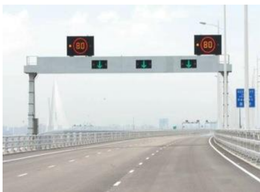
Variable speed signs
